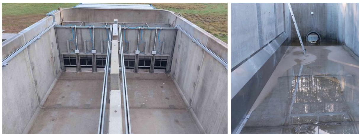
Fig. 1. A reservoir with a system of installed sluice gates to flush the tank. Visible line of installed supports for wide tanks (without walls). On the right, installed walls separating the recipient track from the supports.
