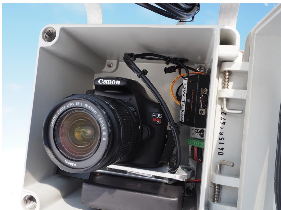
Fig. 31. Internal view of the Harbortronics system.
