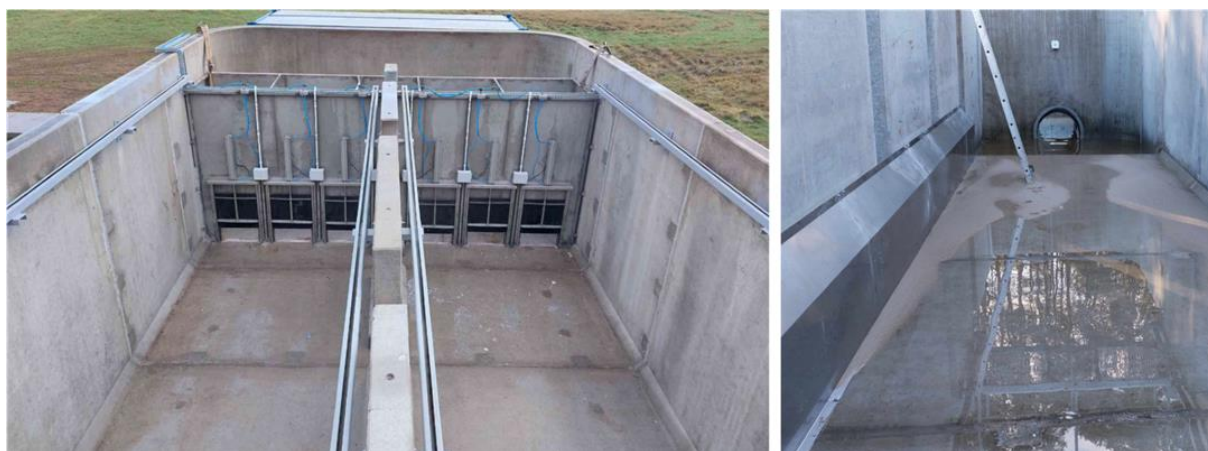
Fig. 1. A reservoir with a system of installed sluice gates to flush the tank. Visible line of installed supports for wide tanks (without walls). On the right, installed walls separating the recipient track from the supports.
